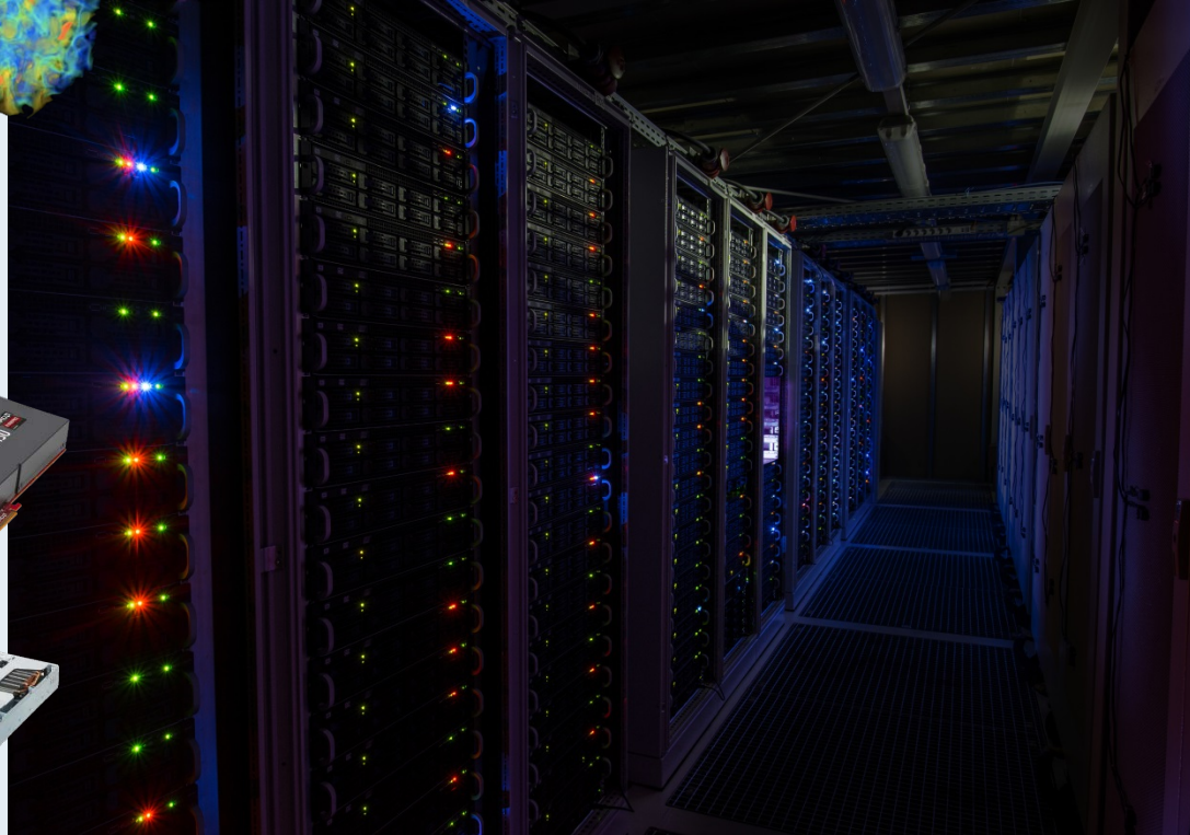
Green DataCenter at GSI, Darmstat, Germany
